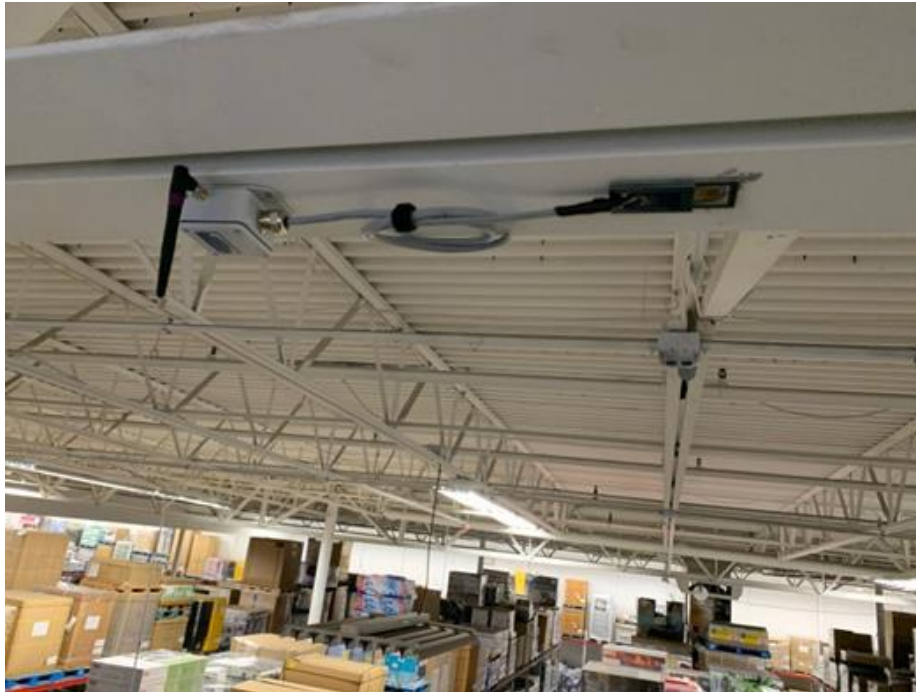
Wireless Strain gauge SenSpot™ at a roof system of a building
