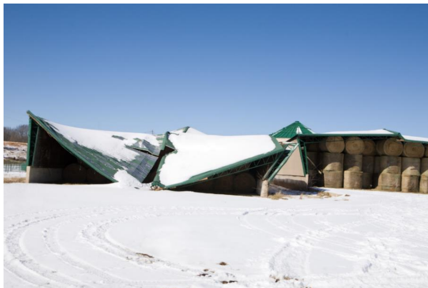
Roof's failure under snow loads
