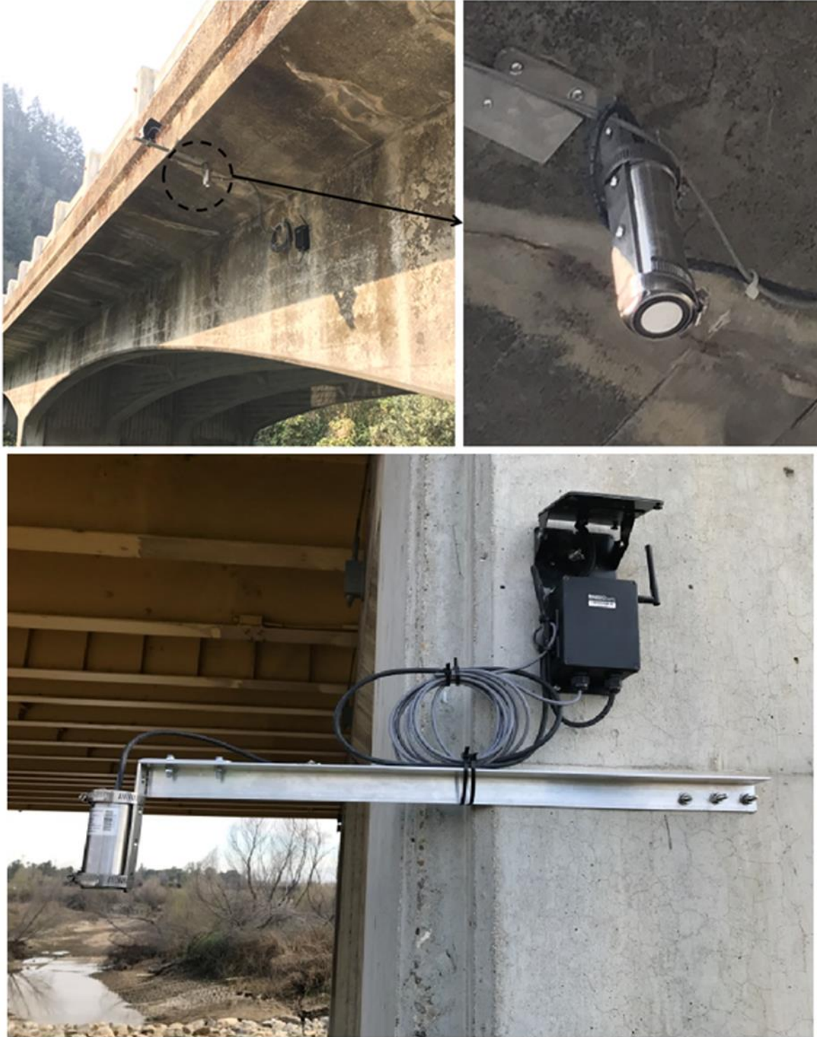
An ultrasonic wireless water level sensor and cameras used for monitoring flood condition on a number of bridges in California
