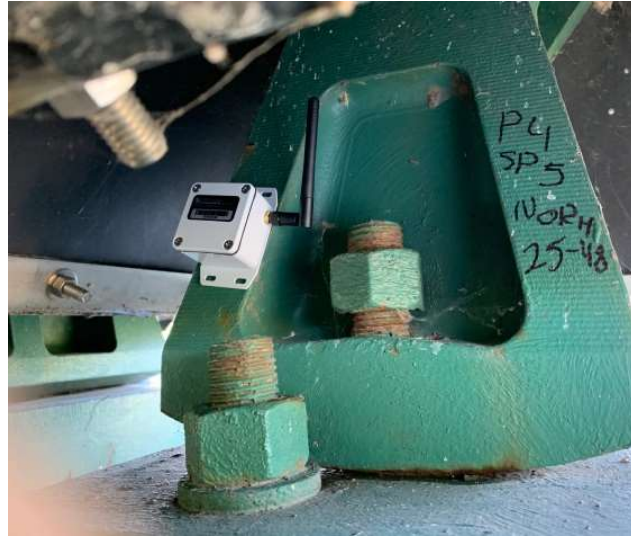
Resensys Wireless Tilt SenSpot™ sensor on bridge bearings to verify and validate FEM models
