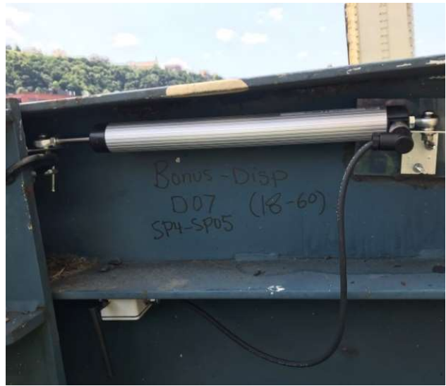
Resensys Wireless Displacement SenSpot™ sensor on bridge expansion joint to verify and validate FEM models
