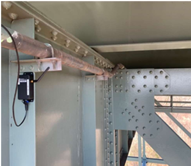
Resensys Wireless Vibration/Acceleration SenSpot™ sensor on a abutment for FEM model verification and validation
