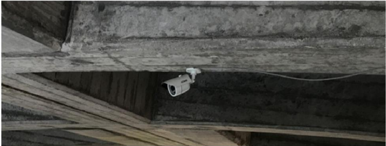
Wireless solar powered cameras used on California and Pennsylvania scour critical bridges.
