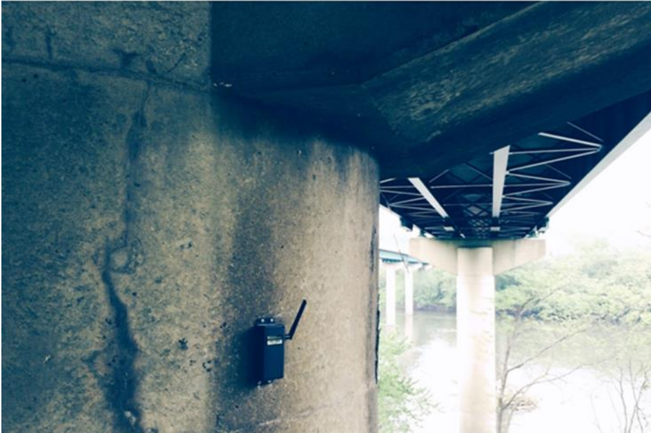
A scour critical I-81 bridge across the Potomac River is monitored using Resensys wireless tilt meters.
