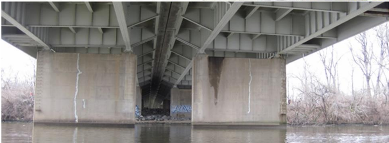
In Washington DC, the bridge on the East Capitol Street across the Anacostia River is monitored using Resensys system
