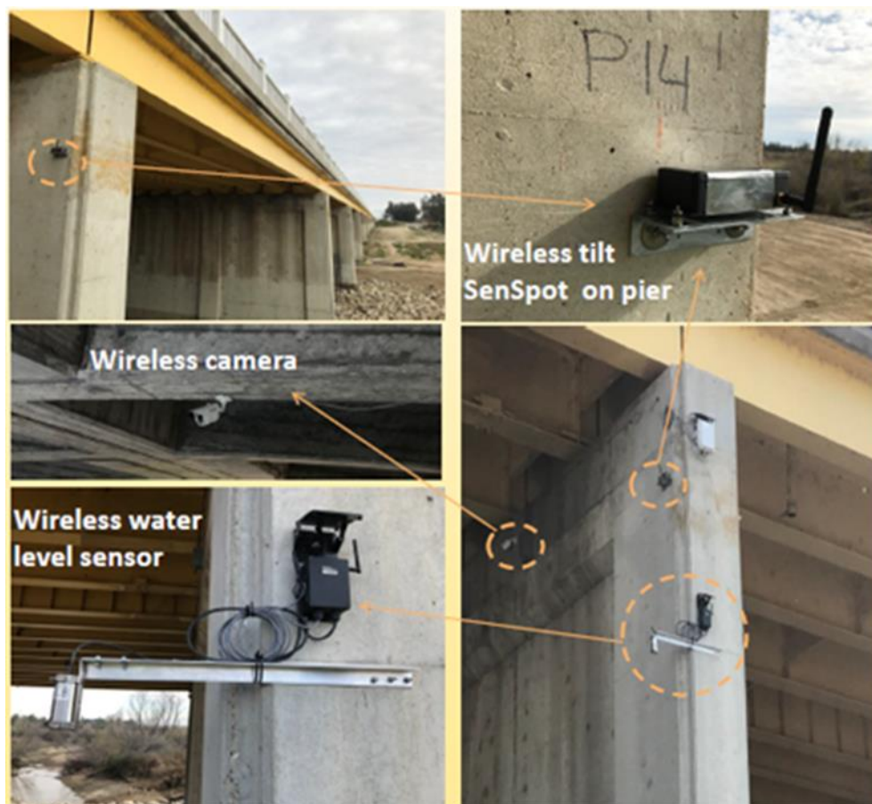
Resensys Wireless Tilt SenSpot™ sensor, Resensys Wireless Water Level SenSpot™ sensor and Wireless Solar Powered Camera on scour critical bridge
