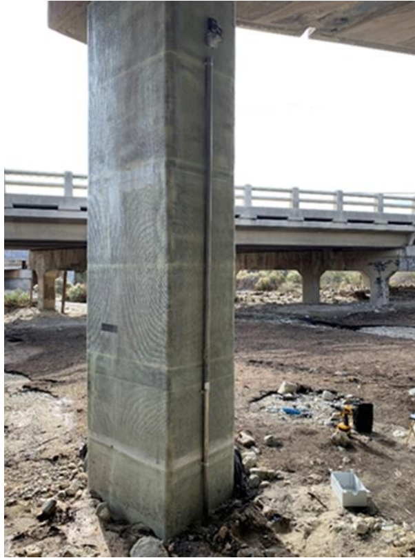
Wireless Scour Probe SenSpot™ sensor on pier of scour critical bridge to measure sediment level
